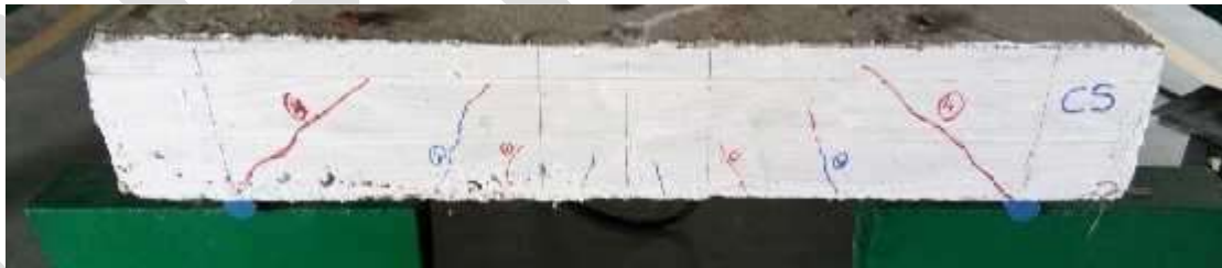
Fig 9. Crack pattern for control specimen
